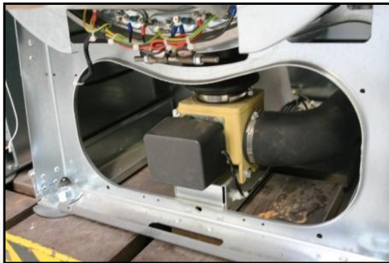
Drain under tub
